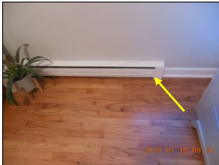
Electric heater did not work
