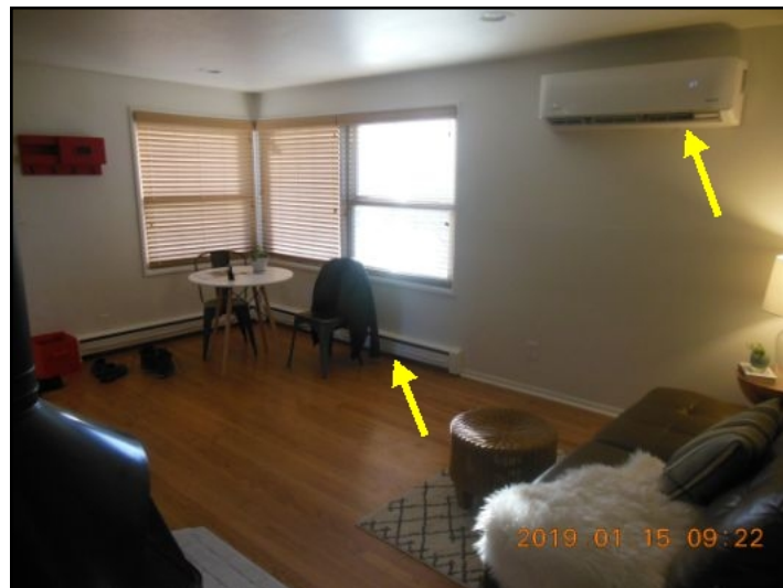
Heat pump and baseboard electric heater in living room
