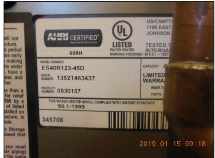
Water heater 6 years old
