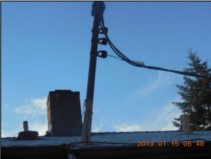
Service mast is not secured
