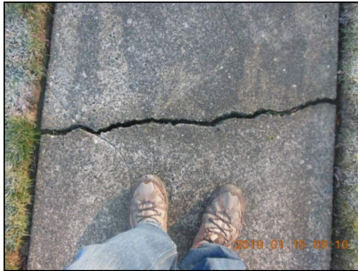
Large crack on walkway
