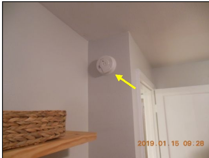
Smoke detector in north side bedroom, but absent in master bedroom
