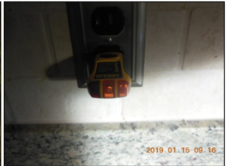
Countertop Outlet without power
