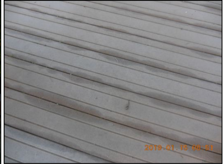
Composite decking boards installed upside down
