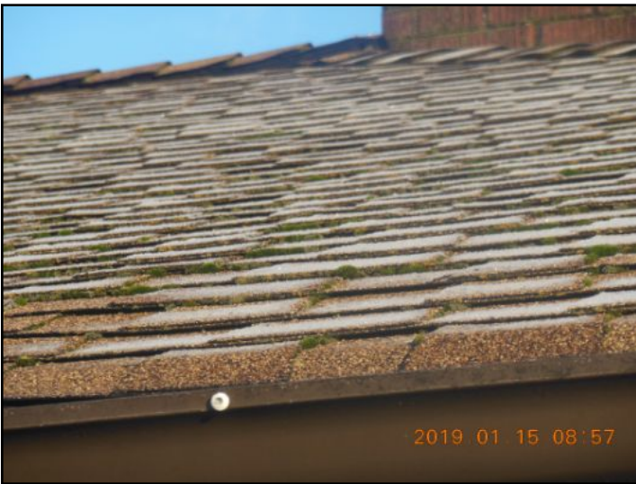
Moss on roof
