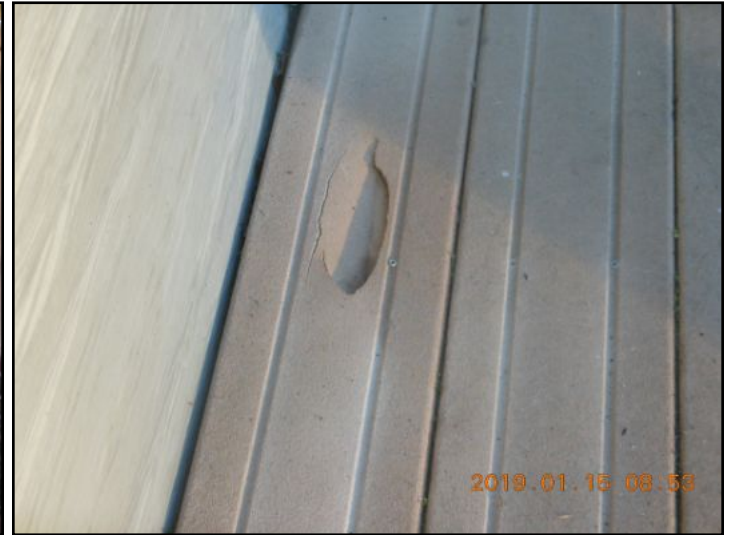
Broken deck board, front
