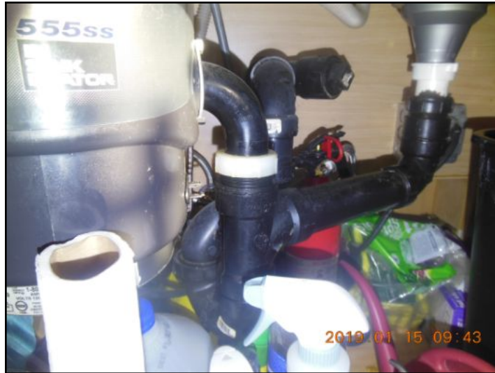
Drain trap too deep
