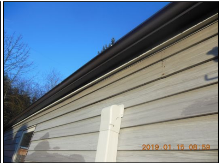
No roof ventilation in the back side
