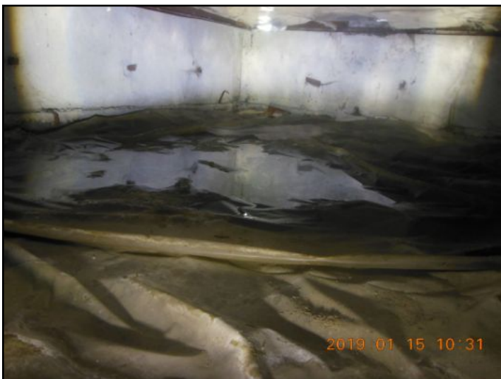
Water puddle in crawl space
