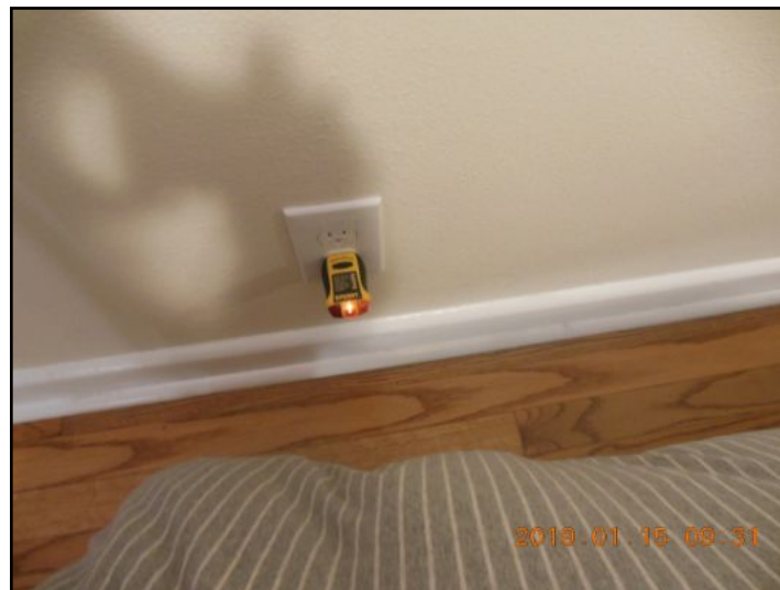
Ungrounded outlets in bedrooms
