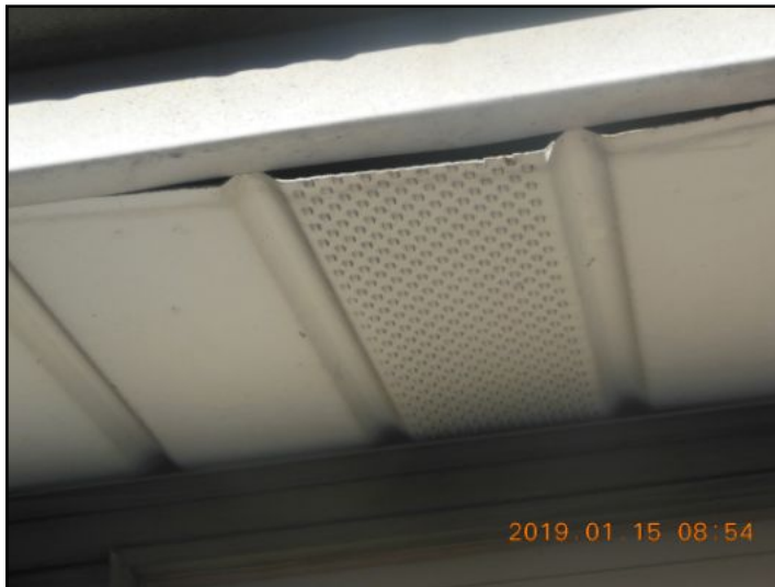
Metal soffit vents loose, minor correction needed
