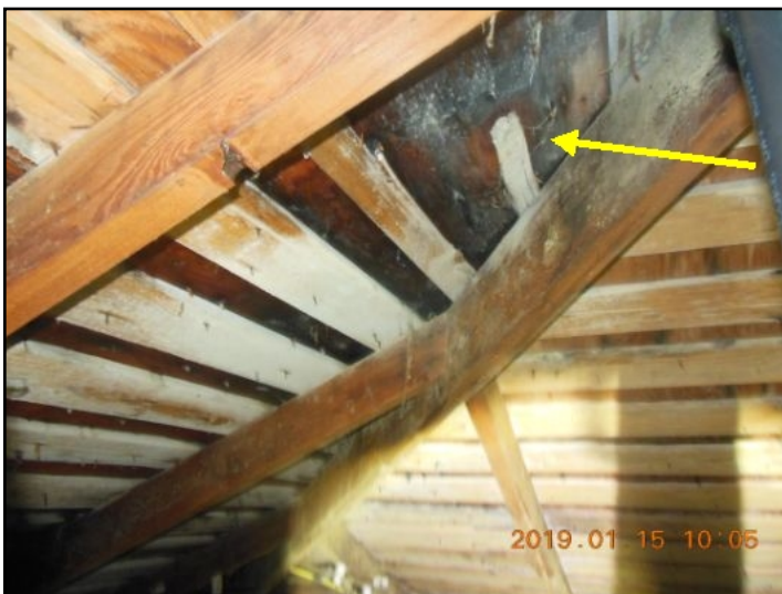
Broken sheathing board and past leaks
