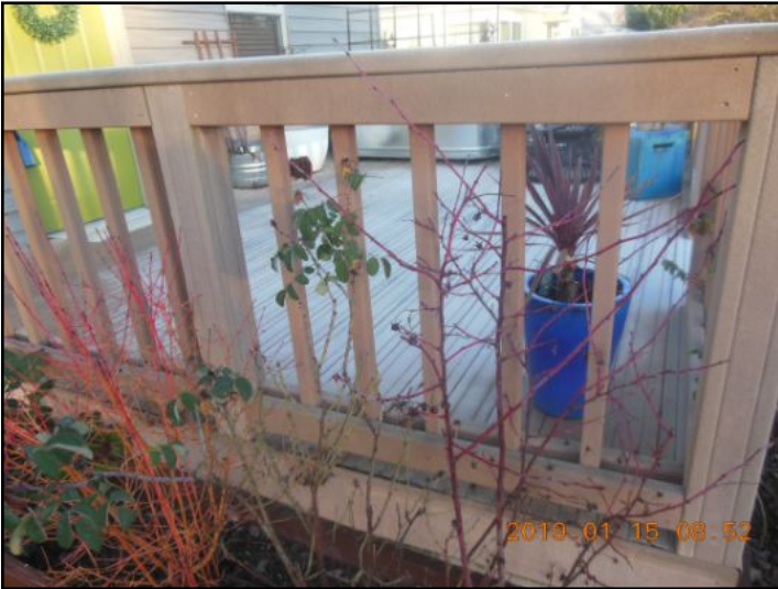
Balusters are separated >4"
