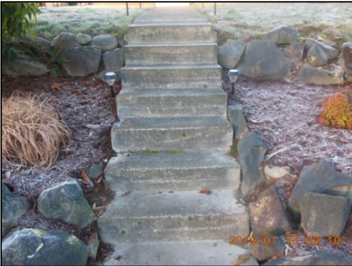
Front steps need handrail
