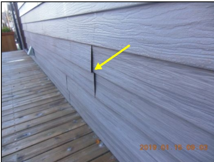
Siding gaps open
