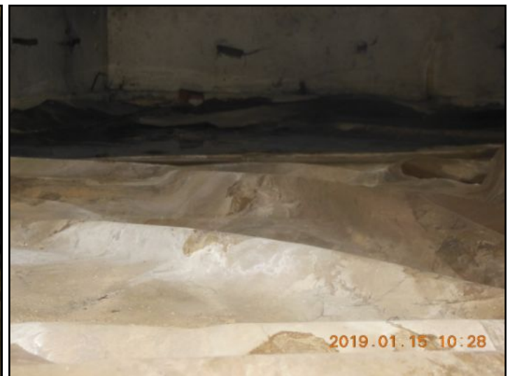
Wrong type of vapor barrier
