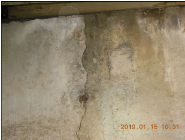
Large crack on foundation wall
