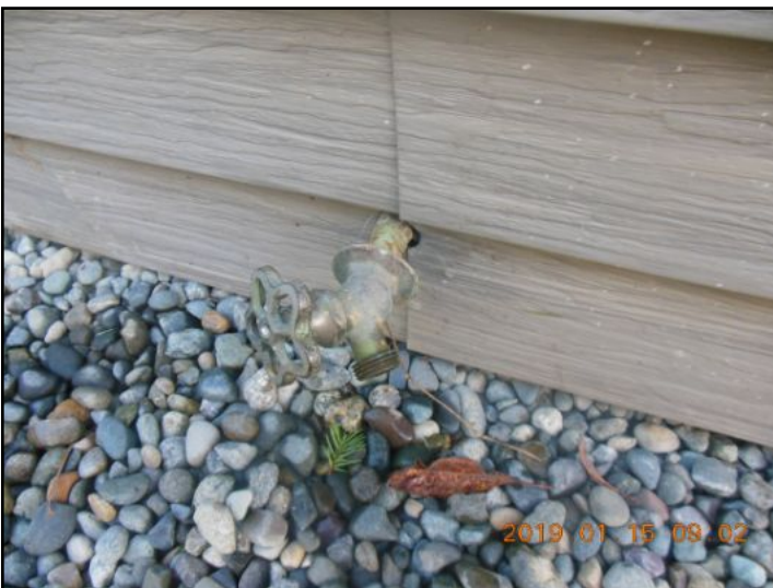
North side faucet- not frost proof
