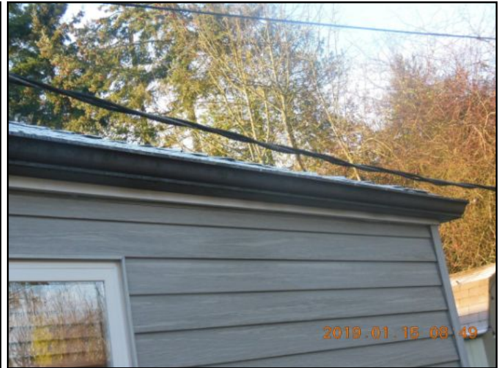
Service drop too close to roof
