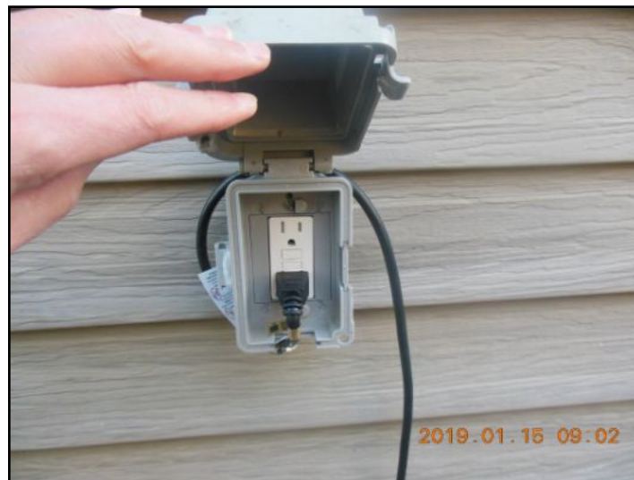
Outdoor GFCI outlet
