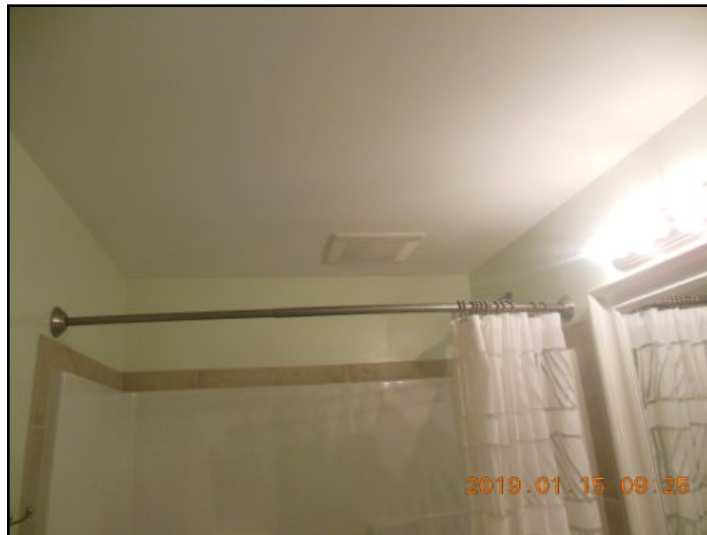
Ceiling and exhaust fan
