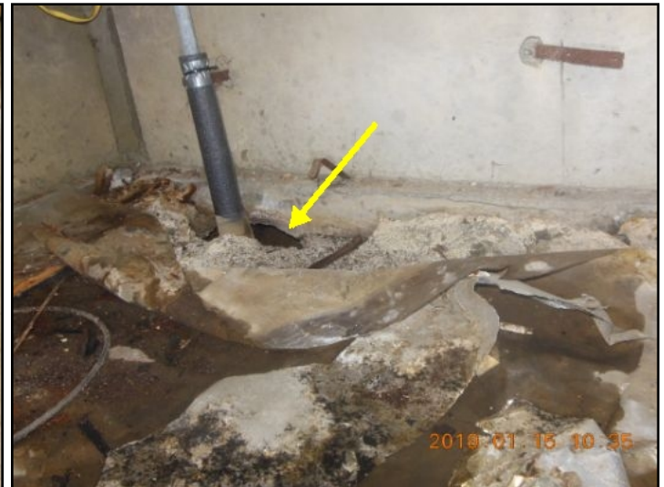
Water puddles and large hole under foundation footing
