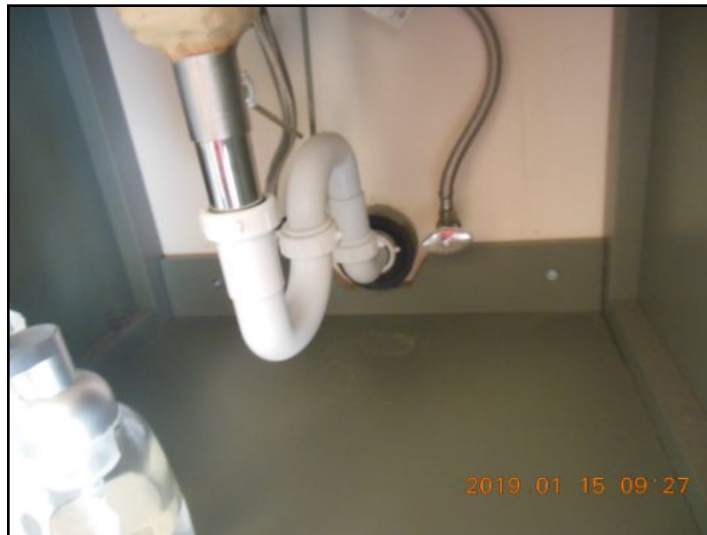
Improper S trap plumbing under bathroom sink
