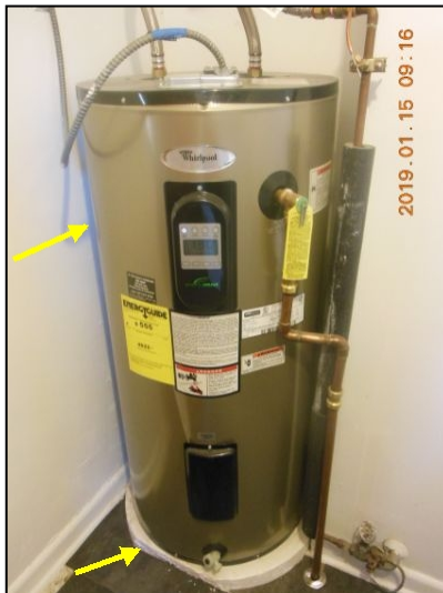
No earthquake straps and no drain pan
