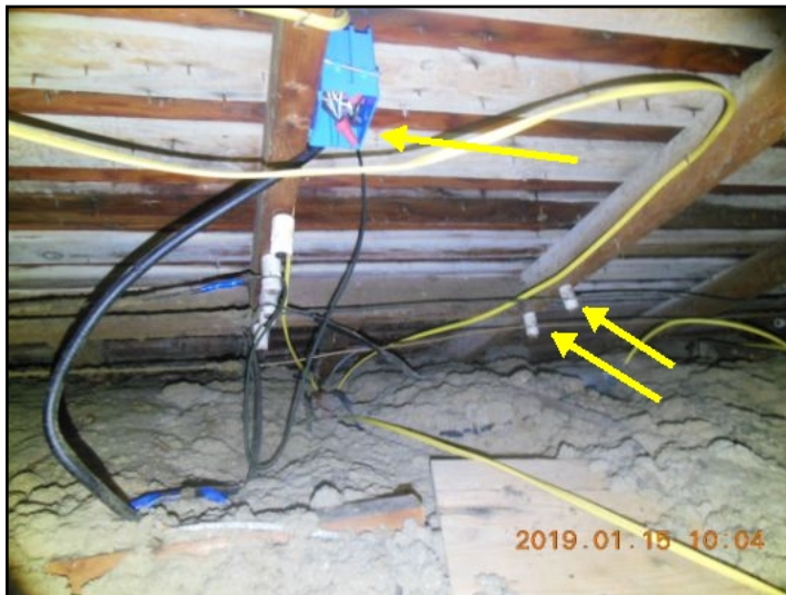
Knob and tube wiring and missed junction box cover
