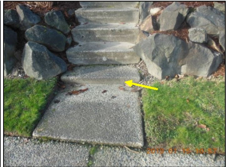
Uneven rise of step may be a tripping hazard
